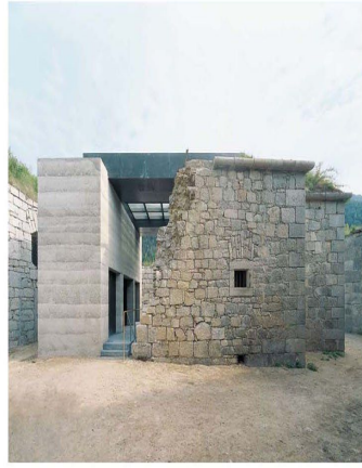
The entrance pavilion combines the new glass construction with the existing partially deteriorated stone-well enclosure. Pumpkiner Area Rider
